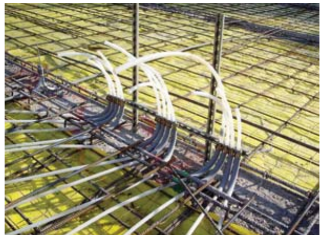
Nathan Hale High School features radiant heating in parts of the building.
